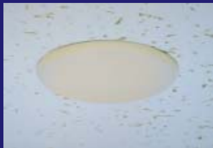
A concealed sprinkler - this is all you see!
